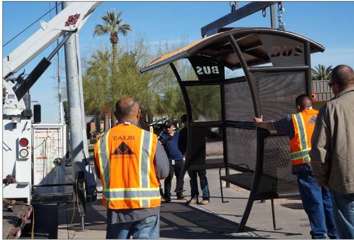
Workers install a new bus shade structure. More than 200 were installed in FY 2019.
