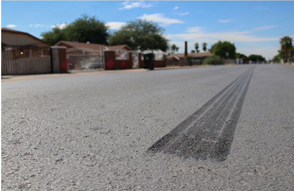
The light gray asphalt sealant is meant to reflect sunlight away from roads to reduce heat, but tire marks like this are one of the aesthetic drawbacks. (Photo by Mingson Lau ( https://cronkitenews.azpbs.org/people/mingson-lau/ )/Cronkite News)
