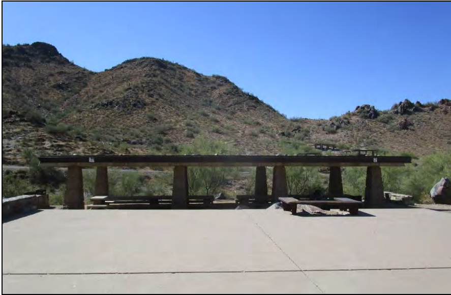
Figure 4. Photograph of Building 5A, a 60-capacity ramada at Building Group 5. View facing south.
