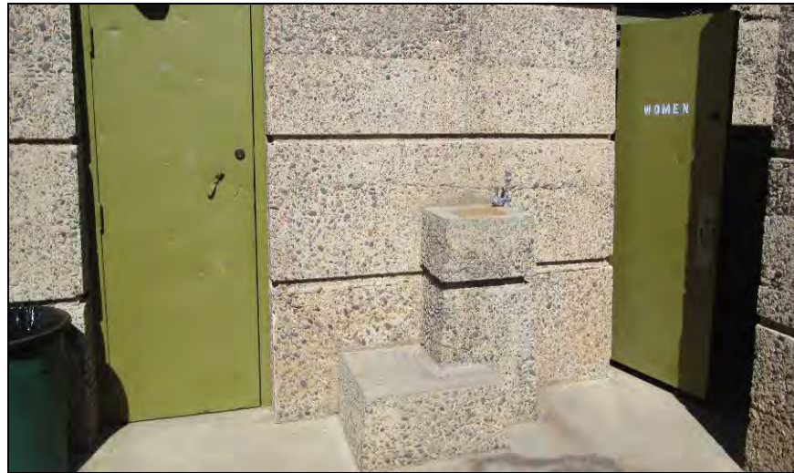
Figure 2. Photograph of the drinking fountain built into the front façade of Building 8, a restroom facility. View facing west.
