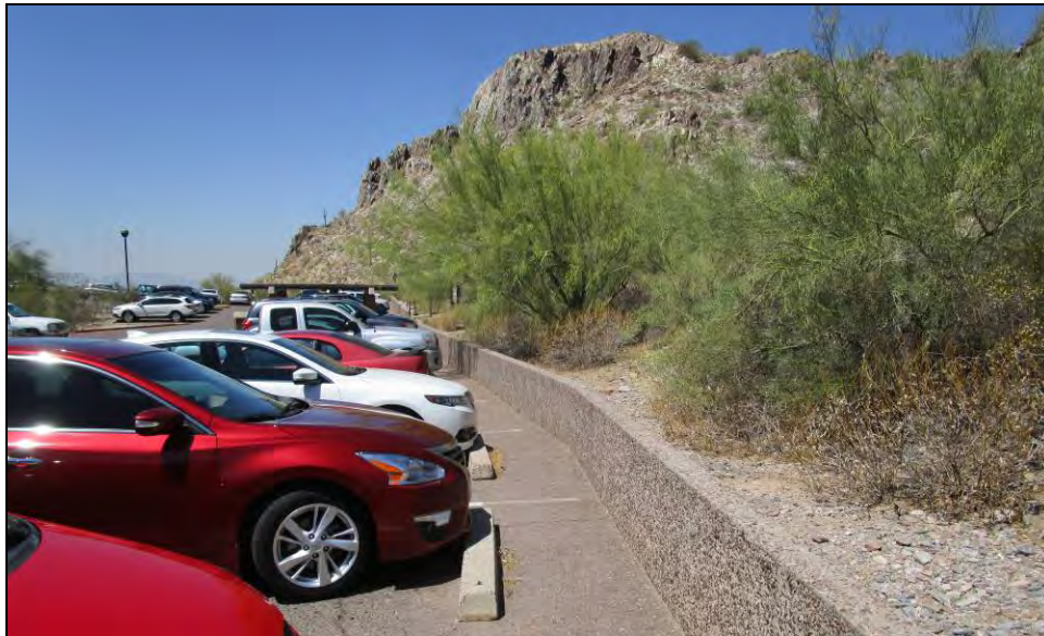
Figure 2. Overview of the retaining wall in the parking lot of Building Group 1, view facing west.
