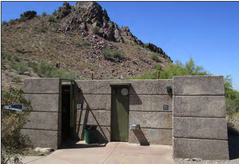
Figure 4. Photograph of Building 2E, a restroom facility of Building Group 2, view facing southwest.
