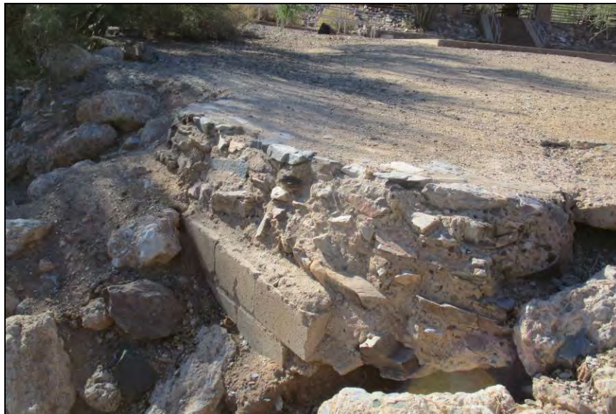
Figure 5. Photograph of a modern retaining wall along the edge of a slope at Building Group 6, view facing north.
