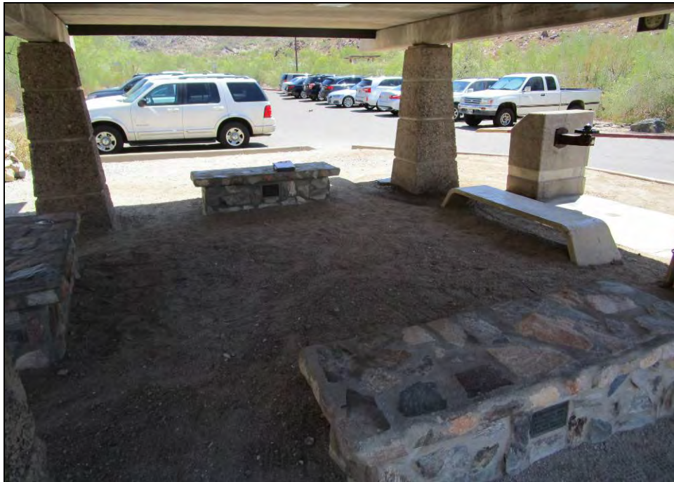
Figure 1. Modern benches under the ramada of Building Group 1. The concrete water fountain is also in view. View facing east.
