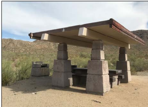
Photograph of a small ramada and concrete barbeque at Five-Tables recreation area, South Mountain Park. View facing southwest.
