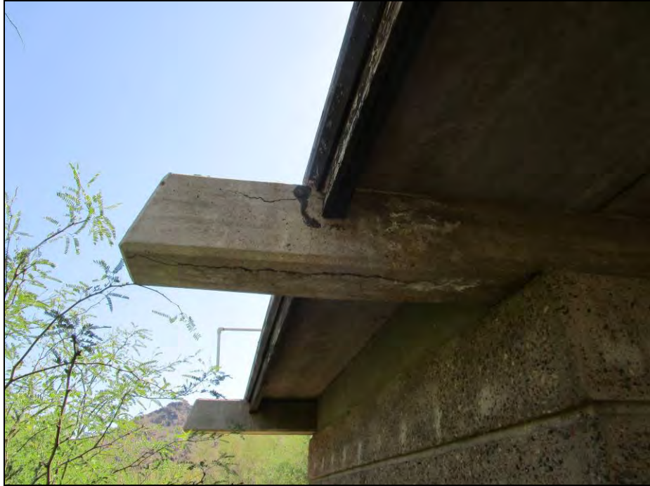
Figure 2. Photograph of the rear façade of Building 3, the Ranger Station, showing condition issues with roof supporting crossbeams. View facing east.
