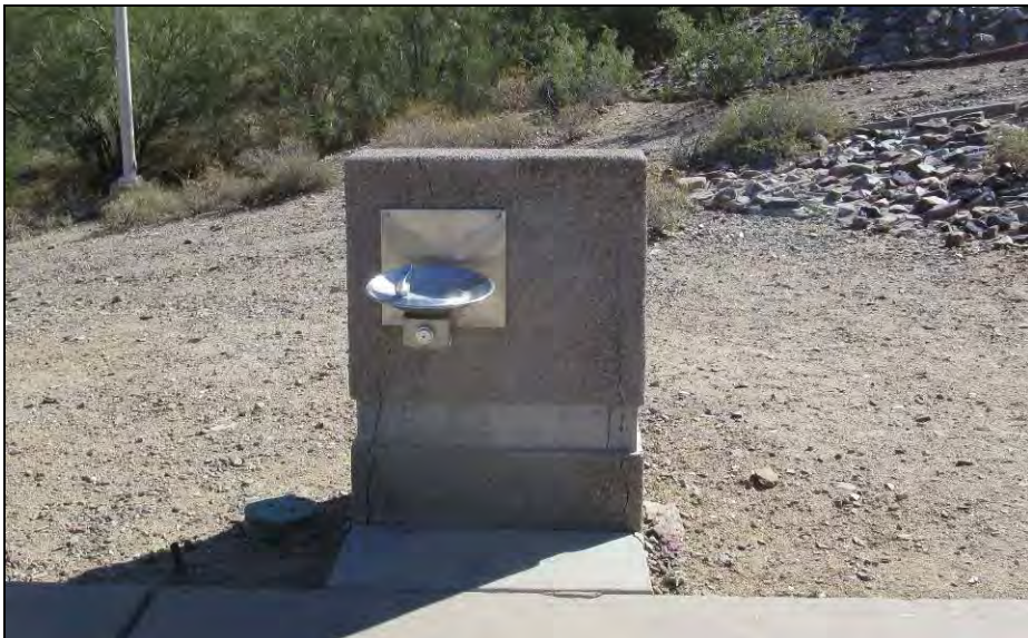
Figure 3. Drinking fountain at Building Group 4, view facing east.
