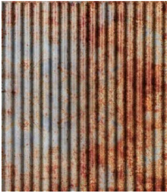
Rusted steel panels
